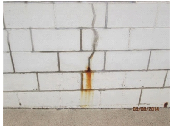
Exterior Surface: Concrete block vertical crack with rust.
