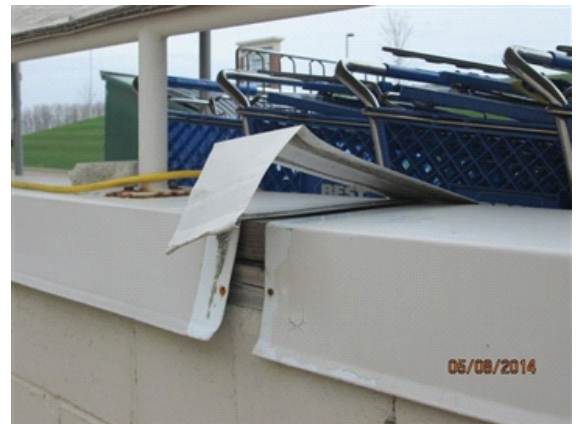
Fences / Enclosures: Top cap is damaged on the loading dock retaining wall.
