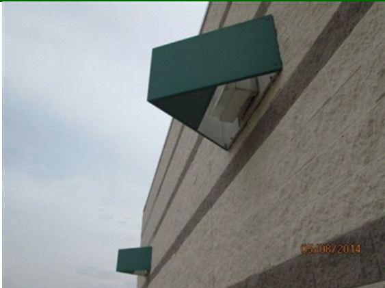
Exterior Lighting: Wall mounted lighting at the front of the building.
