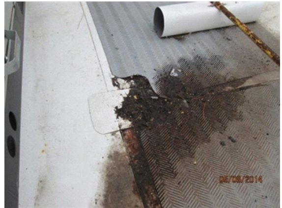
Roofing: Dirt has settled in the ponding area.
