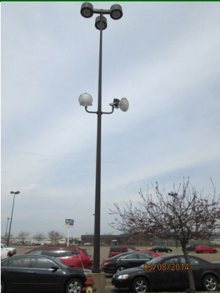
Exterior Lighting: Pole mounted lighting in the parking lot.
