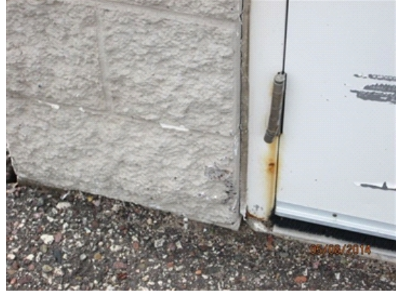
Freight Doors: Rust at bottom of service door.
