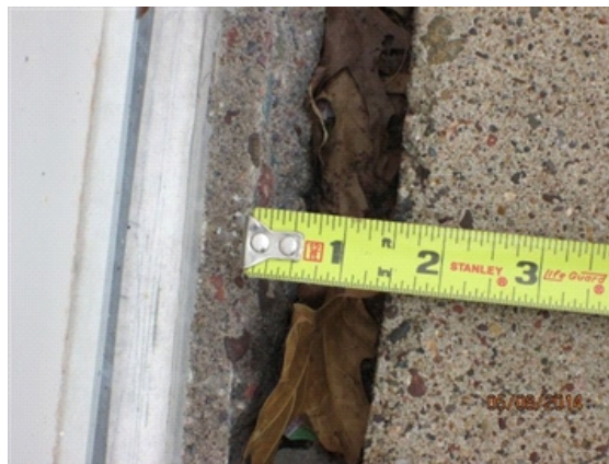
Flatworks/Sidewalks: Sidewalk has pulled away 1.5" on the east side of the building.
