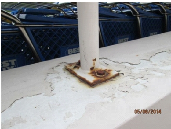
Fences / Enclosures: Rusted bolted connection of railing on top of loading dock wall.
