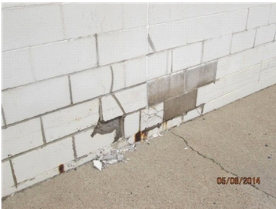
Exterior Surface: Deteriorated concrete block face.
