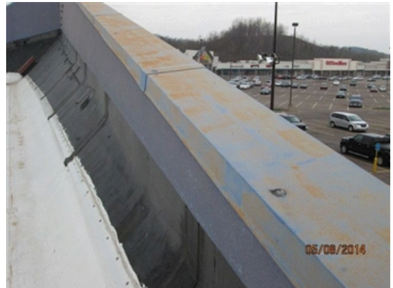
Roofing: North side galvanized top cap flashing that is showing signs of rust.
