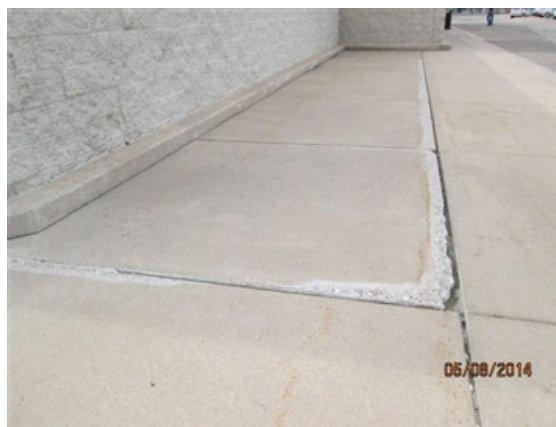
Flatworks/Sidewalks: Sidewalk at front of store showing signs of settlement. Has edges ground down.
