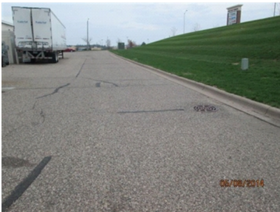
Grading / Drainage: South side of property. Adjacent property is at a higher elevation.
