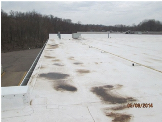
Roof Drainage System: View of the roof's south edge looking west. Gutter is to the left side.
