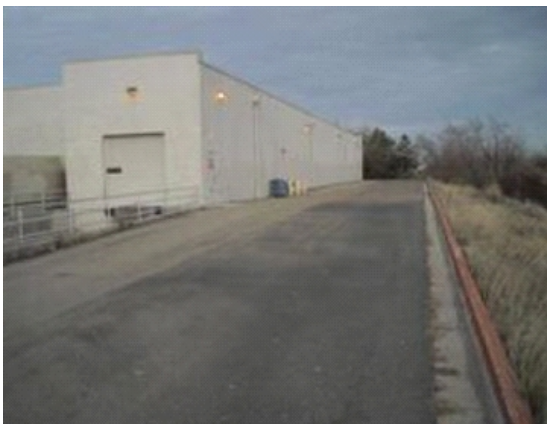
Grading / Drainage: South side of property. Adjacent property is at a higher elevation.
