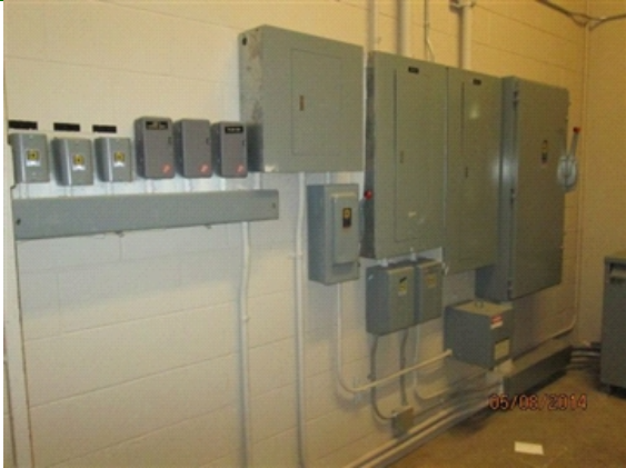
Electrical: Secondary electrical distribution room.
