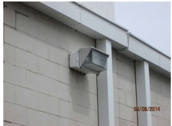
Roof Drainage System:
