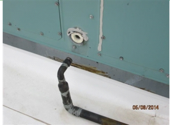
Draft Control/Vent: RTU - 7 condensate line is disconnected from unit.
