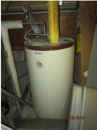
Water Heater: Water heater above ceiling space.
