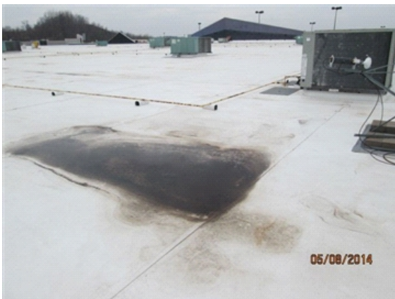
Roof Drainage System: Area of ponding on the roof.
