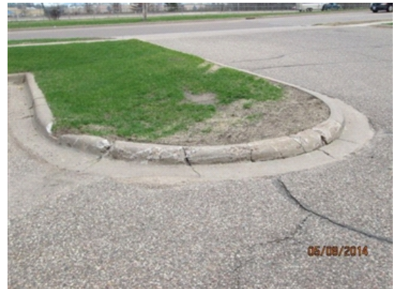
Retaining Walls/Landscaping: Curbing at southeast driveway. Note the 'drive over' area of dead grass.
