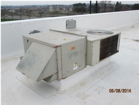
Heating (Carrier units): Smaller Carrier unit.
