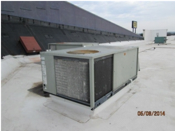
Cooling: Roof Top Unit accommodates both heating and cooling.
