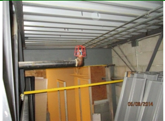
Plumbing: Fire protection system at roof metal decking.
