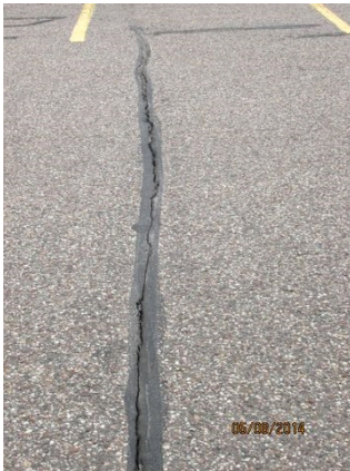
Parking Lot: Larger crack on the east side drive area.
