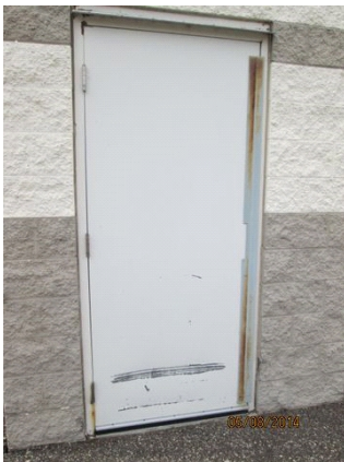
Main Doors: Service door with scratch in the bottom of door and a small spot of rust at base of frame.
