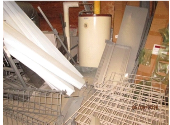
Water Heater: Access to water heater above ceiling space was blocked by stored materials.
