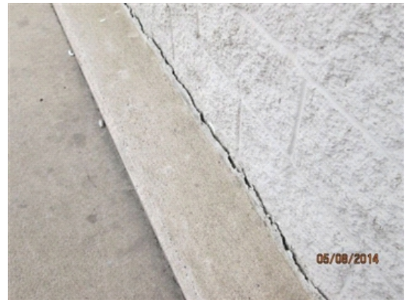
Exterior Foundation: Open joint at foundation wall.
