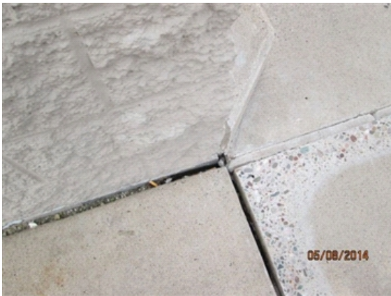
Exterior Foundation: Movement of sidewalks at foundation.
