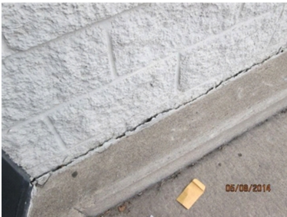
Exterior Foundation: Open joint at foundation wall.
