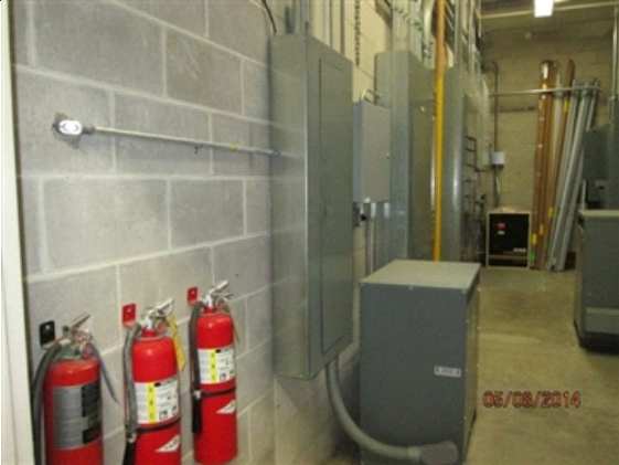
Electrical: Main electrical service room with panels and main disconnect.
