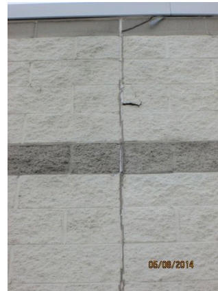
Exterior Surface: Vertical crack in wall extending all the way to the top of the parapet wall where the block has broken.
