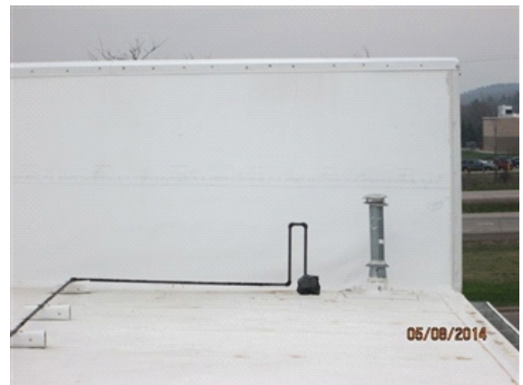
Roof Drainage System: Parapet wall looking east - gutter to the right side of photo.
