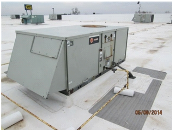
HVAC Distribution: Roof Top Unit - Typical discharge directly into the space below with minimal distribution.
