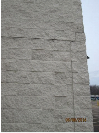
Exterior Surface: Vertical crack in concrete block at corner.
