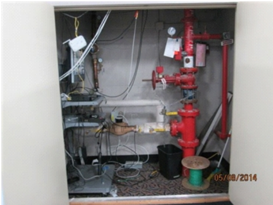
Plumbing: Fire protection and water service closet.
