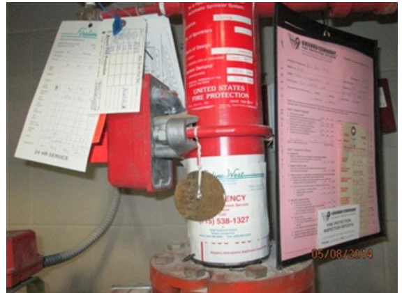
Plumbing: Fire protection service tags and records. All up to date.
