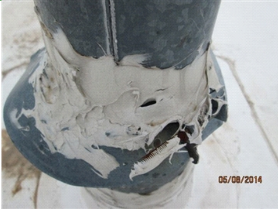
Draft Control/Vent: Open hole in caulking at vent pipe.
