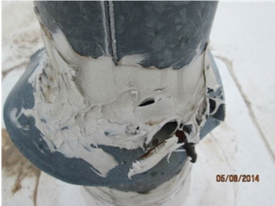
Flashing/Valleys: Open hole in caulking at vent pipe.
