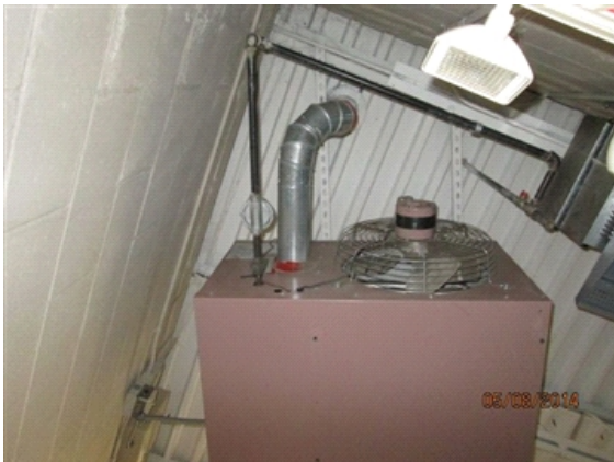
Draft Control/Vent: Gas fired unit heater ventilation through roof.
