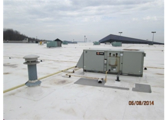
HVAC Distribution: Roof Top Unit and exhaust wiring.
