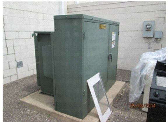
Electrical: South side transformer and meter.
