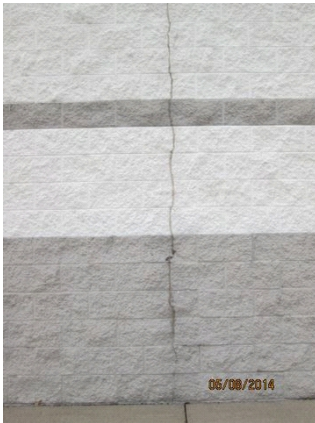
Exterior Surface: Vertical crack in wall.
