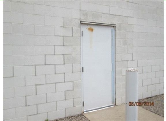
Main Doors: Exterior service door - note spot of rust at top of door.
