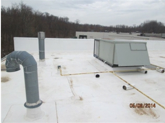
HVAC Distribution: Roof Top Unit and exhaust venting.
