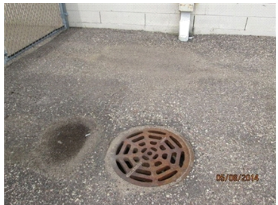
Grading / Drainage: Catch basins on the property take rainwater from the roof through downspouts and underground into the catch basins.
