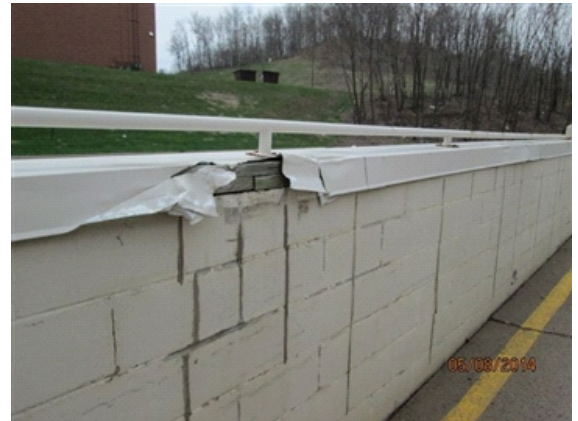
Retaining Walls/Landscaping: Retaining wall damaged top cap and block mortar joints in need of painting.
