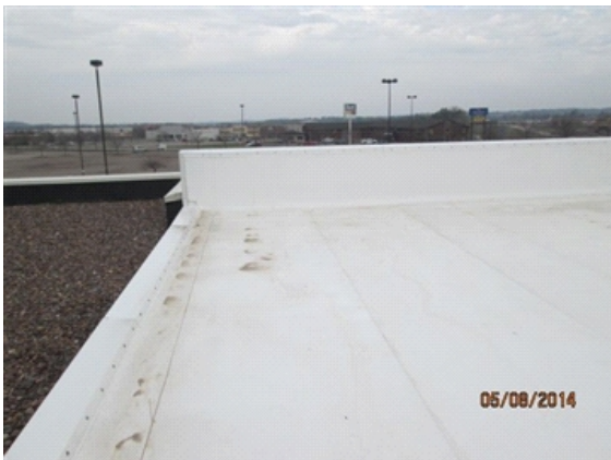
Parapet Wall: Parapet wall looking north along the west side next to adjacent roof area to another store.
