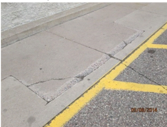
Flatworks/Sidewalks: Sidewalk area that has been ground down to eliminate a tripping hazard.
