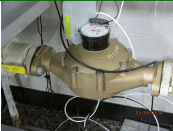
Plumbing: Water service meter located near the fire protection riser in closet off of retail floor.
