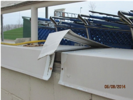
Retaining Walls/Landscaping: Top cap is damaged on the loading dock retaining wall.
