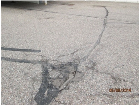
Parking Lot: Parking lot cracks
