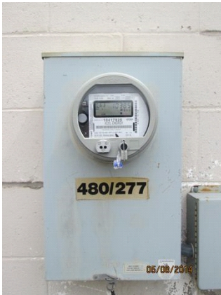
Electrical: Electric meter located on south exterior wall near transformer.
